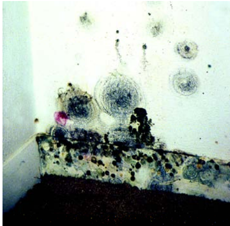
Photo 3A: Mold growing in closet as a result of condensation from room air
