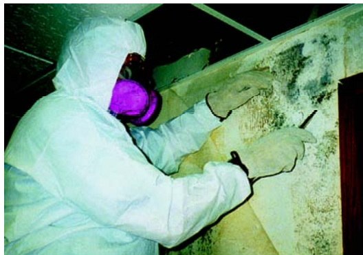
Photo 7: Remediation worker with limited PPE
